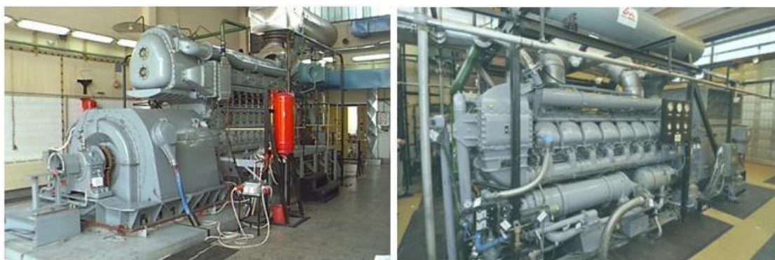
Figure 1-13: The emergency diesel generators of Installations I and II
