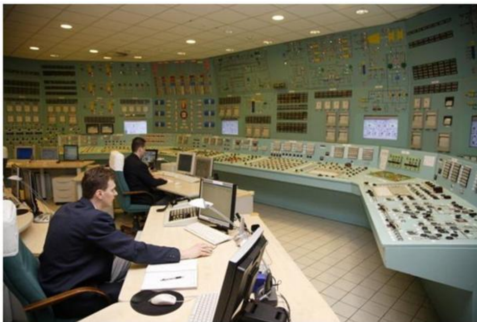
Figure 1-9: Picture of unit control room
