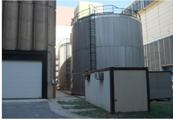
Figure 2-5: Demineralised water tanks of Installation II next to the wall of the service building
